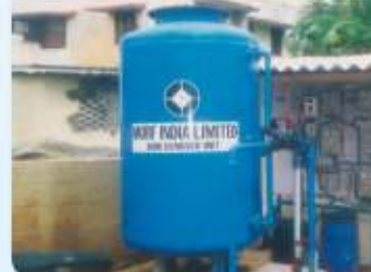
HV Iron Remover with Dosing Pump
