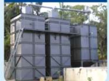
FBBR - Sewage Treatment Plant
